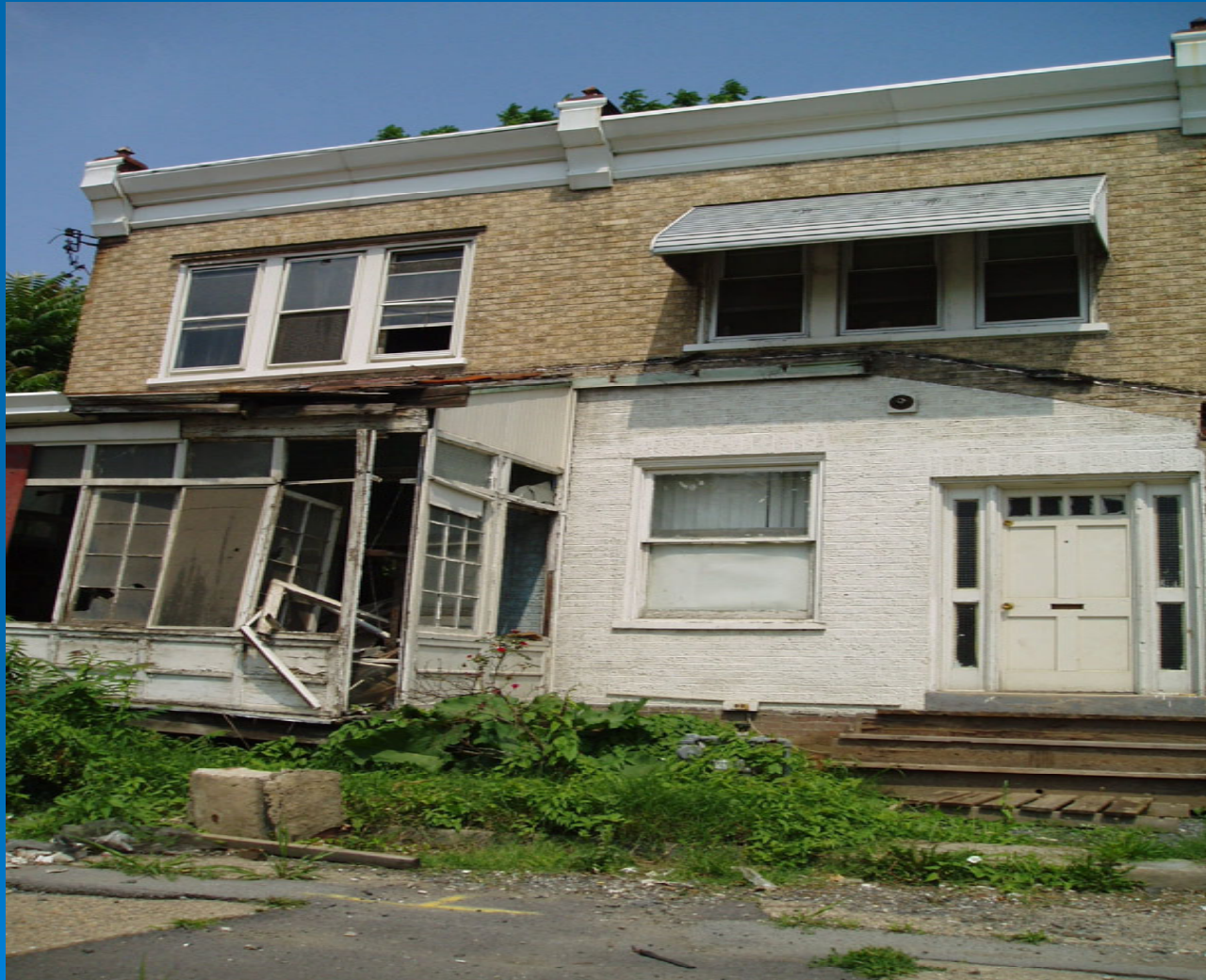
Failing walls; two families may live side-by-side.
